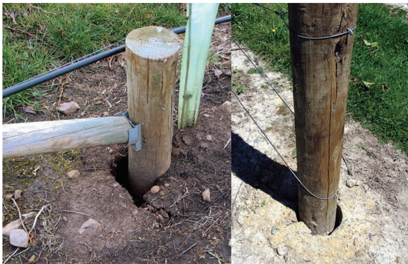
Fig. 6.30. Left: an end assembly post moving in the soil. This could be due to the weakness of recently disturbed soil in this newly developed vineyard. Right: a free-standing end post that is starting to lean into the row. A tieback of some sort is required.
