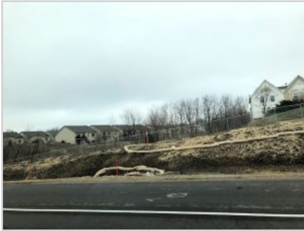
New construction is particularly sensitive to erosion, this disturbed shoulder off of I-35 near Ankeny is using a few techniques to control erosion-straw waddles and straw to help grass seed establishment. Photo Credit: Amber Anderson.
