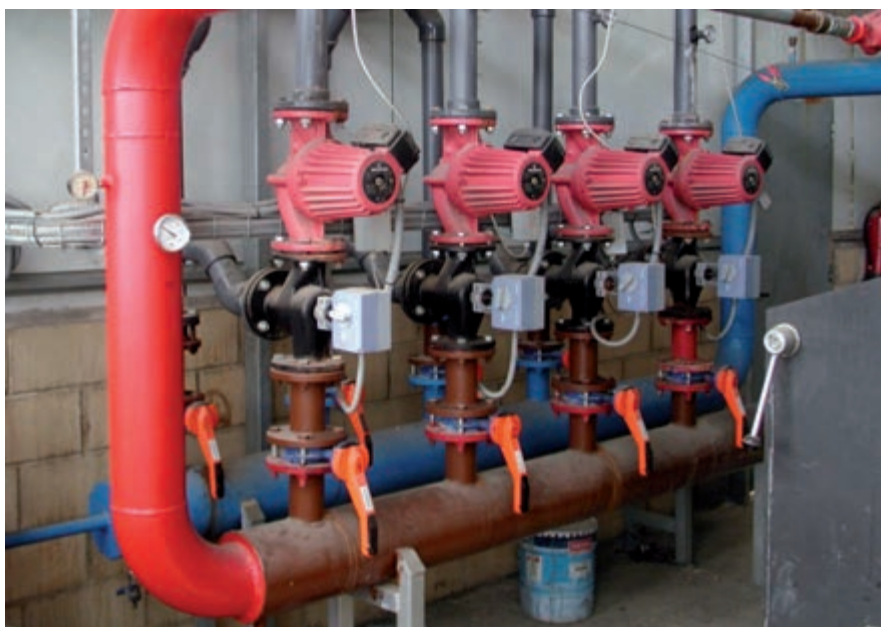
Figure 95. Variable-drive displacement pumps for the distribution of heating water in greenhouses
