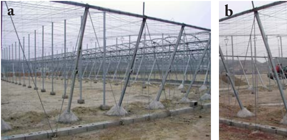
Figure 23. Structure of the lateral band of an Almería-type greenhouse with top perimeter, strap of steel angles and steel stability braces (a), and detail of a direct anchor between two stability braces (b)
