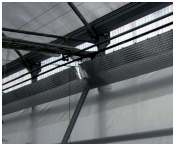
Figure 104. Darkening screen on the side of a greenhouse
