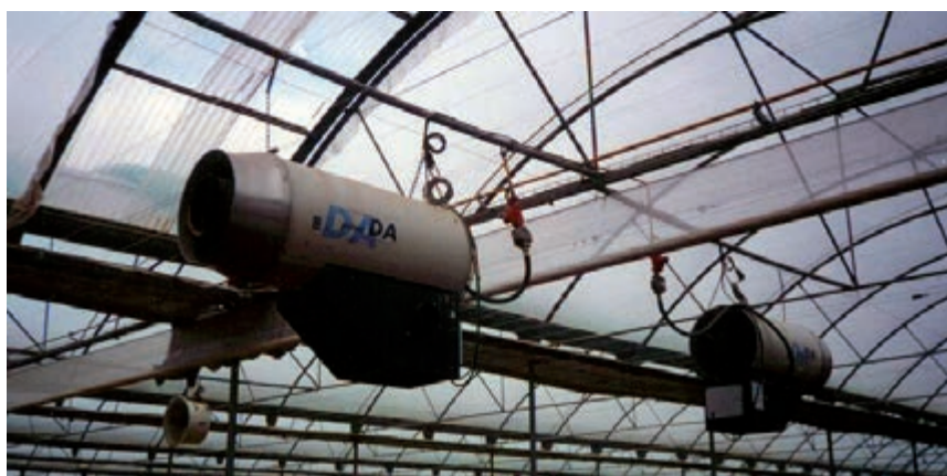
Figure 76. Direct-combustion hot-air generators
