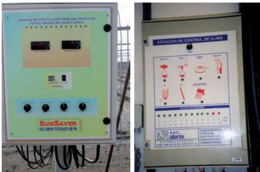
Figure 114. Programmable controllers used in greenhouse climate control systems
