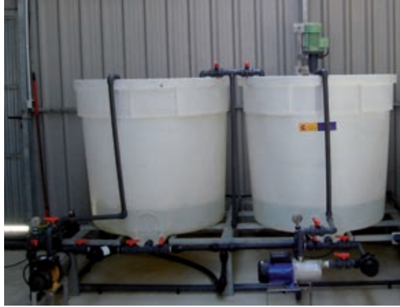
Figure 142. Tanks with agitator system and impulsion pumps of a phytosanitary treatment system using a stationary network of fog systems
