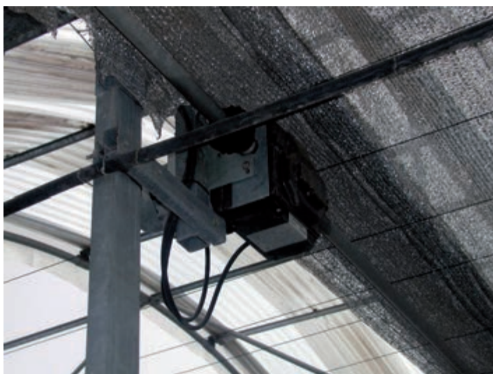
Figure 103. Geared motor that drives the suspended thermal screens
