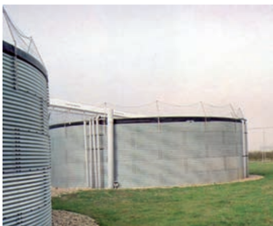
Figure 97. Hot-water storage insulated tanks for heating of greenhouses in the Netherlands
