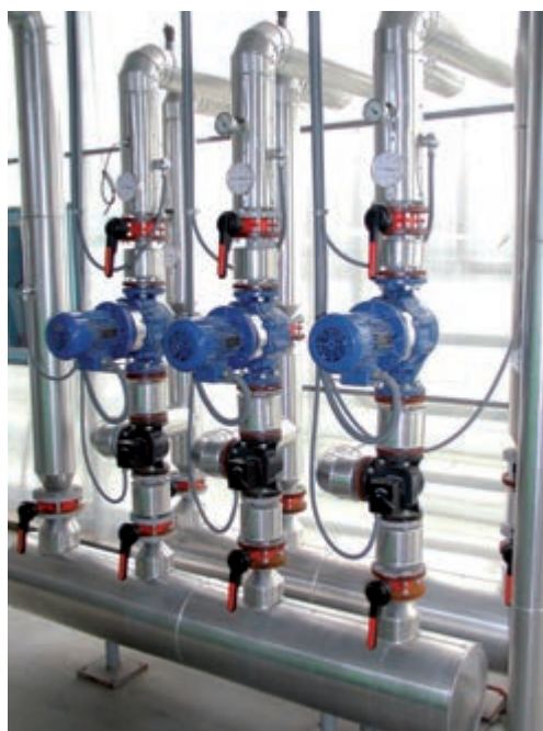
Figure 84. Main piping system of a greenhouse heating system with an insulating covering and three-way valves for temperature regulation
