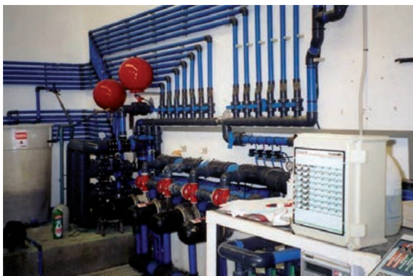
Figure 120. Automated fertigation facility
