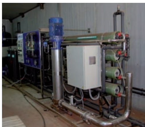
Figure 126. Desalination equipment for well water for use in greenhouse irrigation
