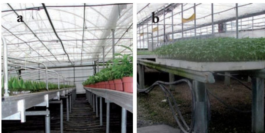
Figure 93. Heating pipes (under seedling trays) resting on the ground (a) and hung from the tables (b)
