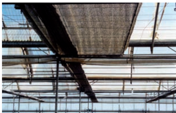
Figure 99. Suspended thermal screen that is retracted in a sector and deployed in the adjacent sector
