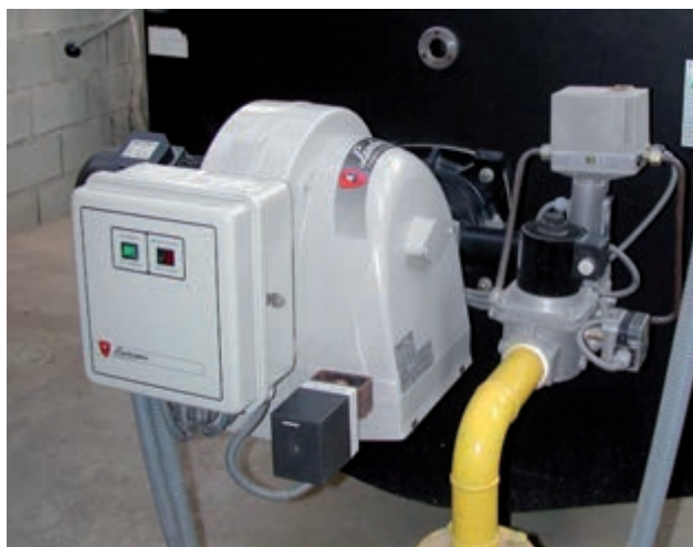
Figure 87. Modulating burner on a boiler for greenhouse heating
