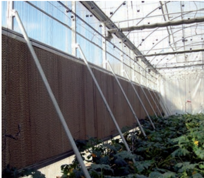
Figure 69. View of a cellulose pad from inside the greenhouse
