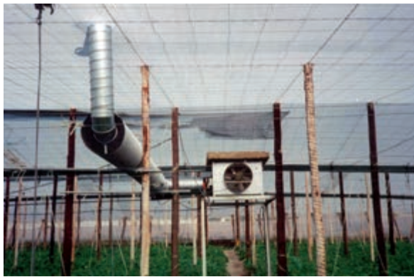
Figure 79. Indirect-combustion hot-air generator in an asymmetrical greenhouse of Campo de Níjar
