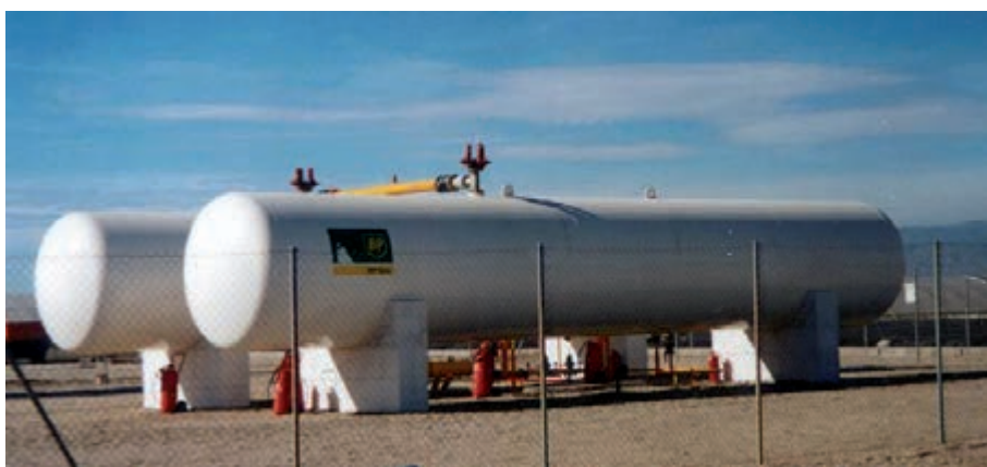
Figure 82. Propane tanks for a heating system
