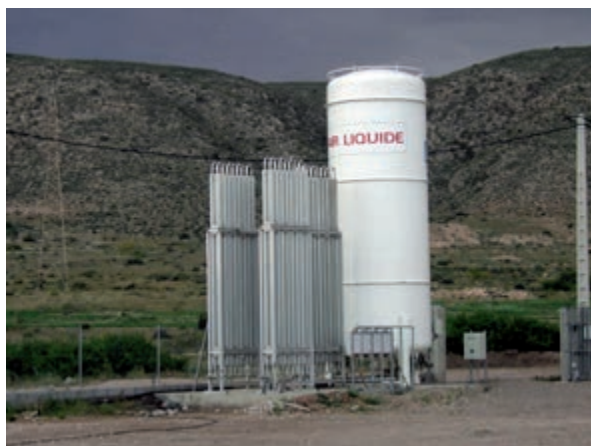
Figure 109. CO 2 tank and evaporator circuits for carbon-dioxide enrichment in greenhouses
