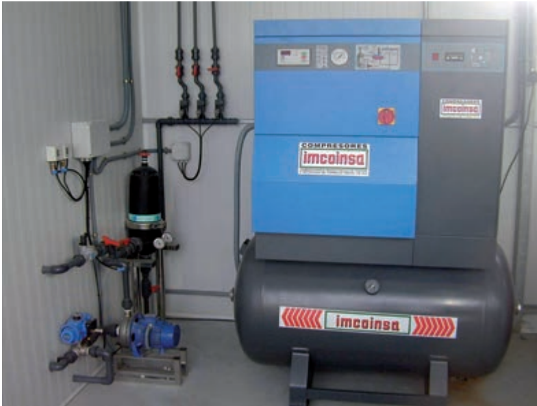
Figure 73. Air compressor and water pump in a fog system
