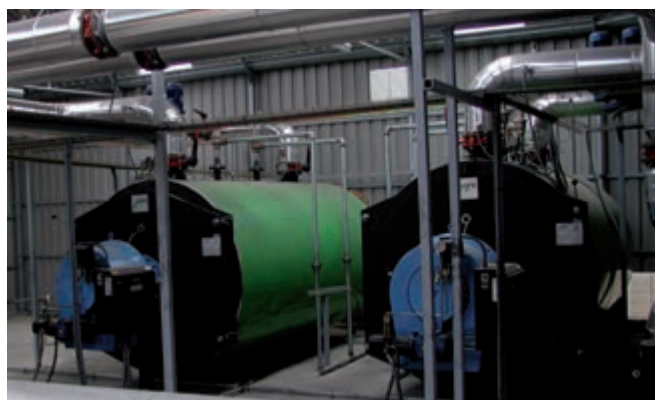
Figure 96. Two-boiler system in Almería greenhouses for hot water generation
