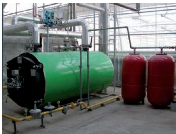
Figure 83. Boiler and expansion tanks in a hot-water heating system in an Almería greenhouse fed by propane gas
