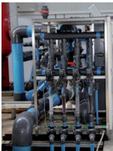
Figure 119. Detail of the Venturi injectors on a fertigation system
