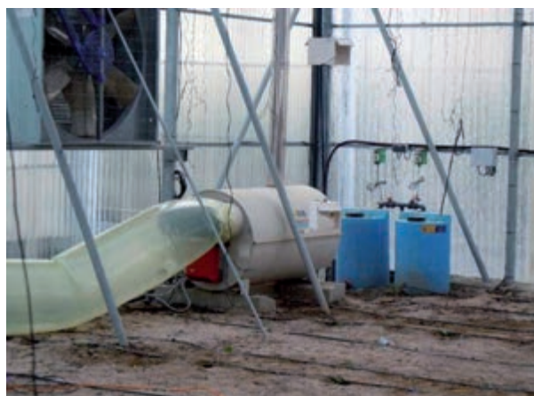
Figure 80. Polyethylene sleeves for hot-air distribution produced by an indirect-combustion generator
