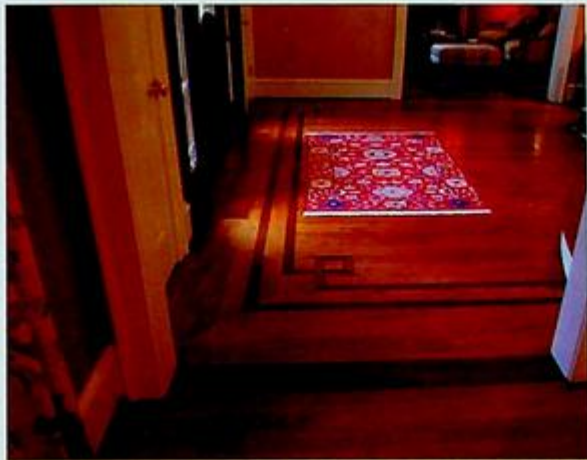
Flush thresholds of sapele, inset into the oak flooring, help separate one room from another. This is a relatively inexpensive detail that can provide an elegant look. The intricate inlays in the foyer are more difficult and more costly.
