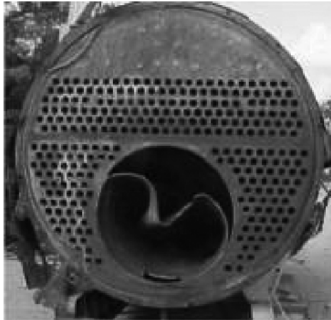
Figure 4. Example of a boiler with the different tubes.
