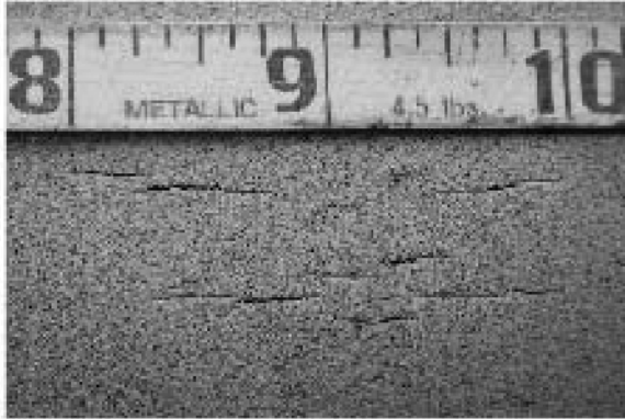
Figure 1. Small “SCC” cracks, that are widespread in tape-coated pipeline.
