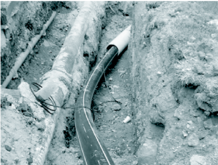
Figure 4. HDPE gas pipe with protective duct being installed close to a drinkable water main and a sewer line.
