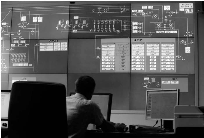
Figure 4.1 Inside the gas storage facility at Incukalns, Latvia. A specialist works in the main control room of Latvijas Gaze’s underground storage facility, August 2014. Photo: Ints Kalnins/Reuters/TT.
