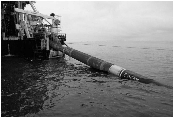
Figure 6.2 Constructing the Nord Stream I pipeline. Poland’s foreign minister Radoslaw Sikorski famously dubbed Nord Stream the “Molotov-Ribbentrop Pipeline”, and other actors criticized the project on environmental grounds. Here the pipeline is being lowered into the Baltic Sea by the Italian vessel Castoro Dieci in summer 2011. Photo: Nord Stream AG.
