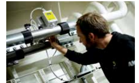
The Air Control unit is installed between the Air Cooler and Feed Doser Valve.
